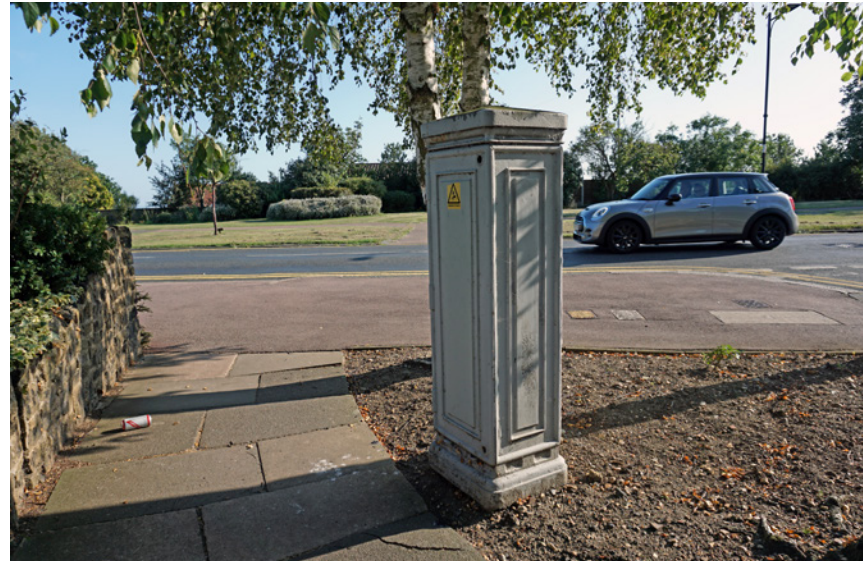
Corporation electricity box
