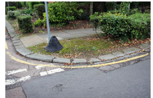
Tarmac road surface in disrepair and damaged granite curbs
