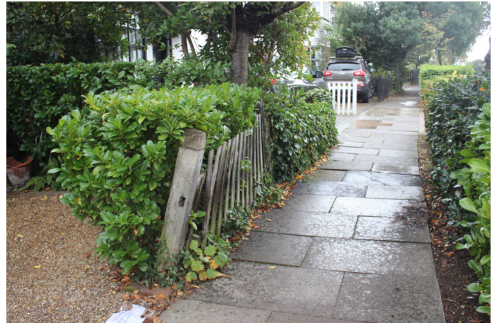
Damaged boundary treatment
