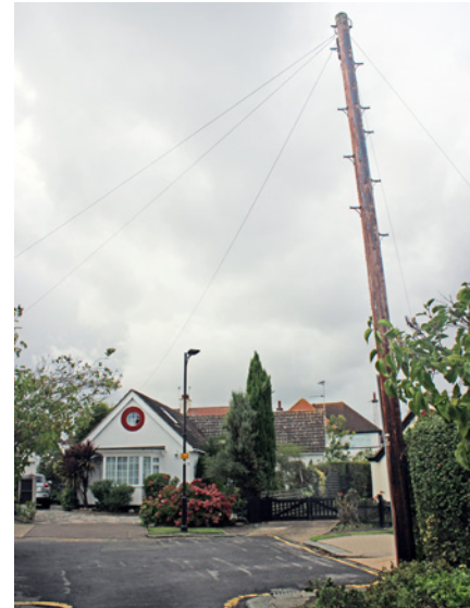
Telephone mast and cables in Ray Close
