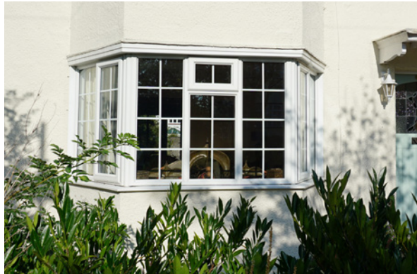
Unsympathetic uPVC window units
