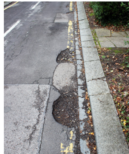
Damage, potholing and patching in tarmac road surface
